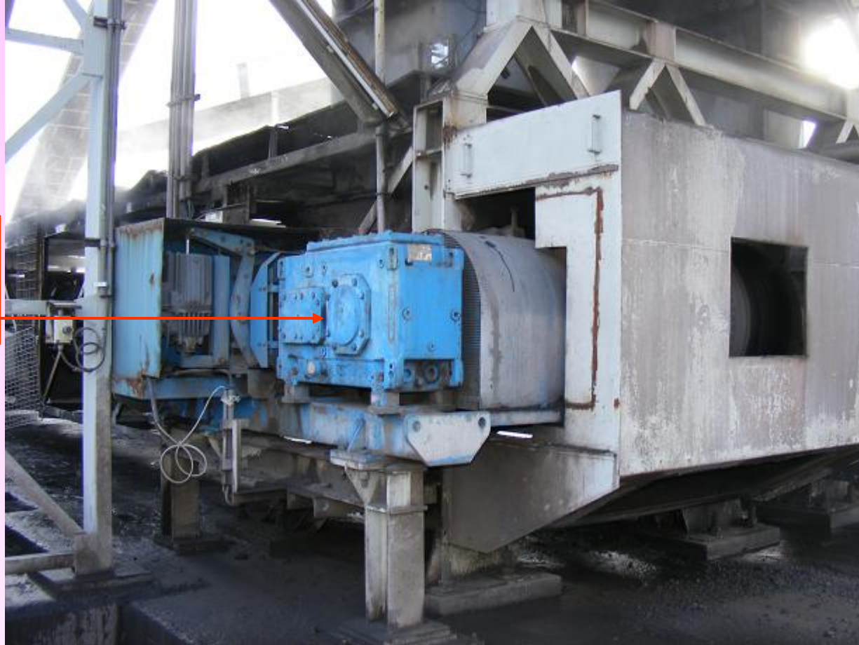
Polytron MTC Gear Box Ash Conveyors System
