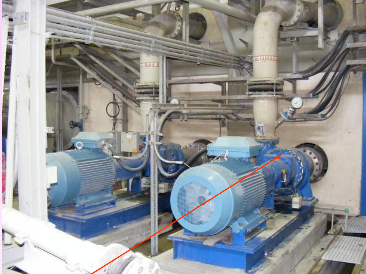
Polytron MTC Bearing – Gypsum Pump F.G.D Plant
